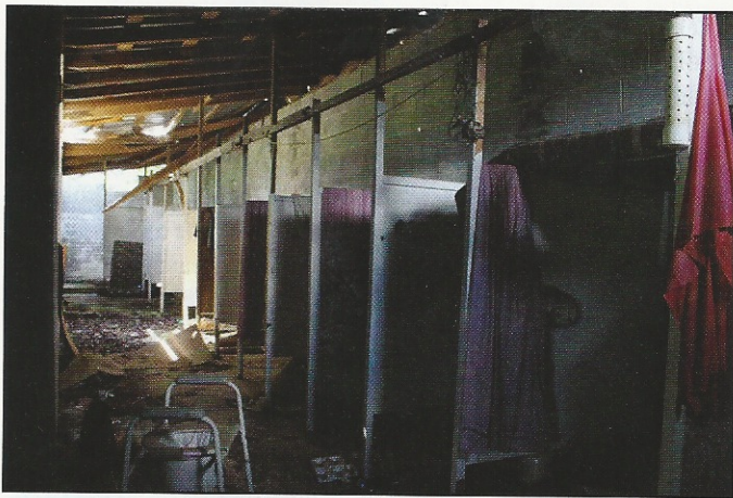
Bathrooms still intact
